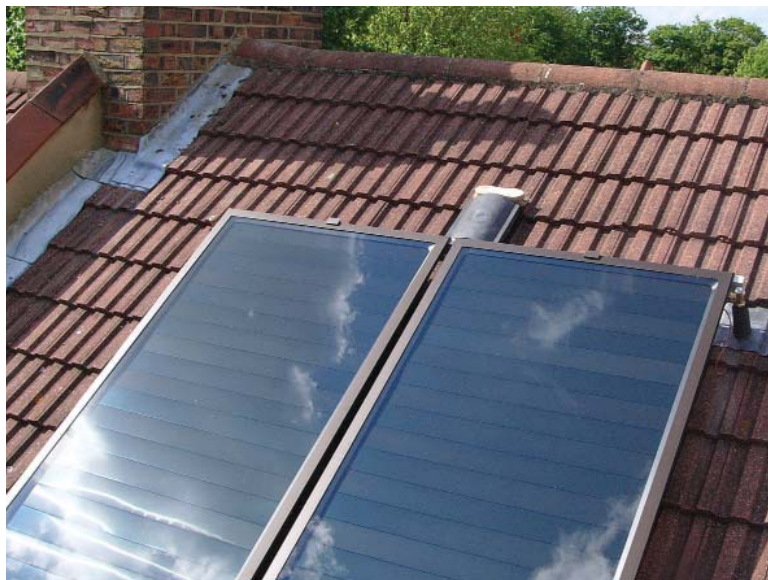
Solar water heating on a roof in Wallington
