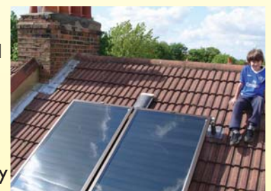
Hot water solar panels on a roof in Wallington
